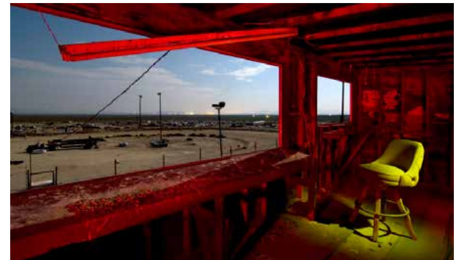
Race Control: While the outdoor portions of the scene of the collapsing press box of the abandoned Pearsonville Raceway in Pearsonville, California have a daylight quality, that look is entirely produced by the long exposure under the light of the full moon. Look in the distance and you can see the city lights along the horizon. The interior colors were painted using a lime and red gelled LED flashlight. The image was made using a Canon 20D, a Tokina 12-24mm (at 12mm), exposed at ISO 100 (3950K) for 120 sec at f/5.6.
